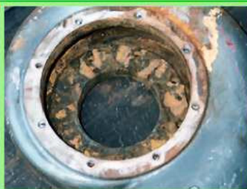
Severe cavitation in pump housing that would normally be deemed scrap
