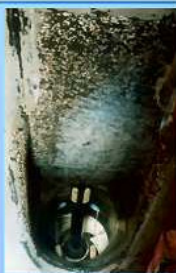
Intake passage showing corrosion adversely affecting water flow
