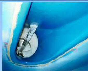
Intake coated which dramatically increases water flow and improves efficiencies
