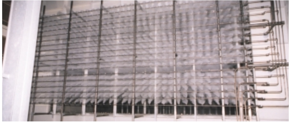
Gas Turbine Mist Cooling System
